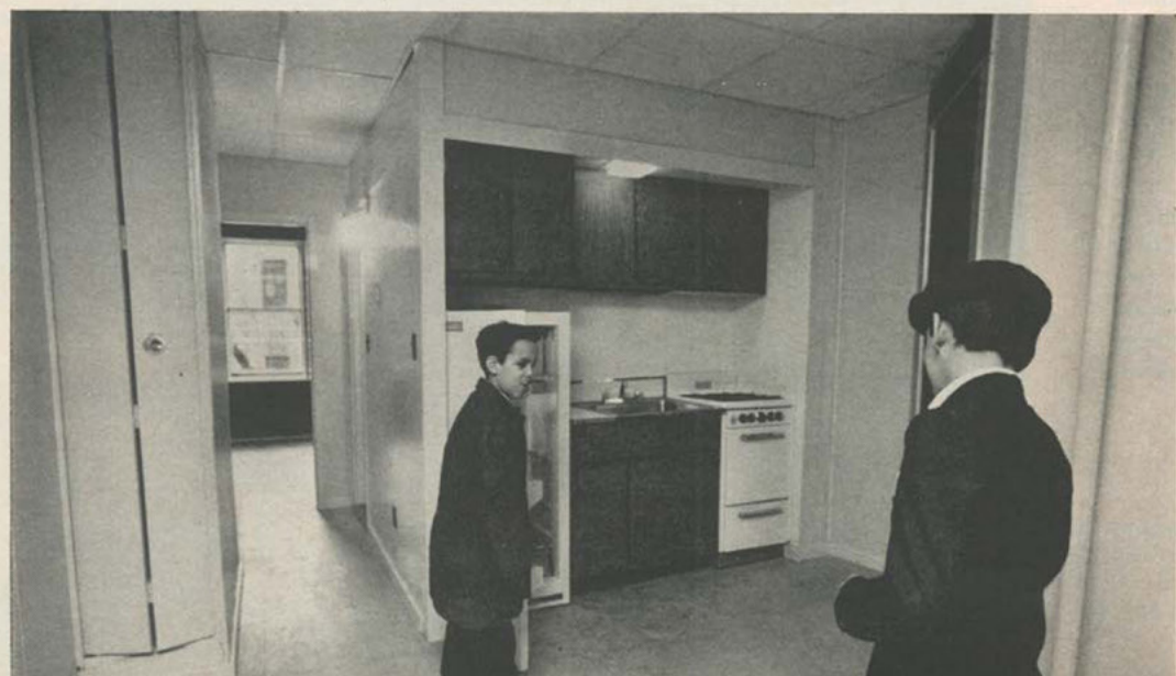
Hector Davila and brother Gregory, 8 (left), examine their new kitchen. In addition to fixing up the apartment, the crew exterminated roaches and rats. The 15 units in the 72-year-old building were completely renovated in 47 hours, 52 minutes—eight minutes ahead of schedule.
